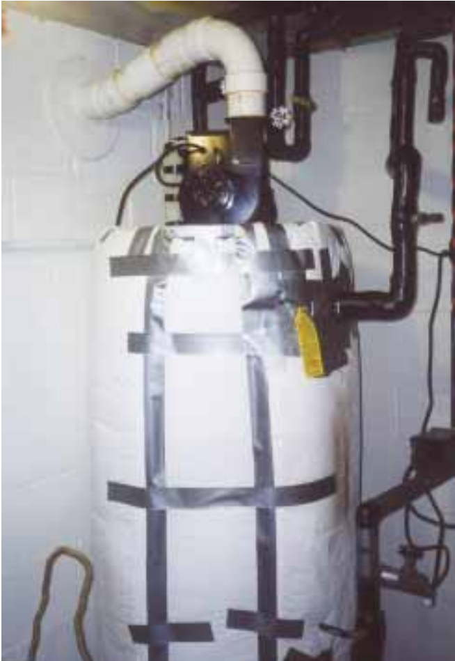
The heavily insulated, backup, natural gas water heater.
