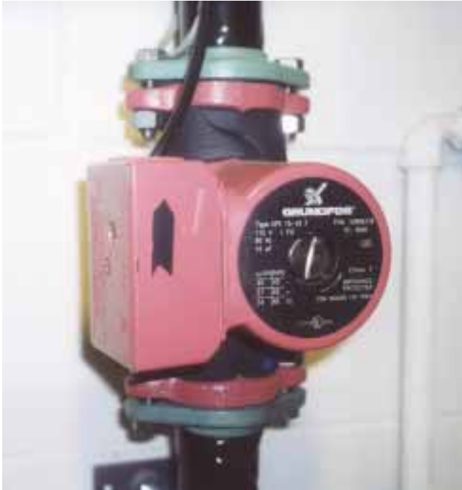
The single, AC powered, Grundfos circulating pump.
