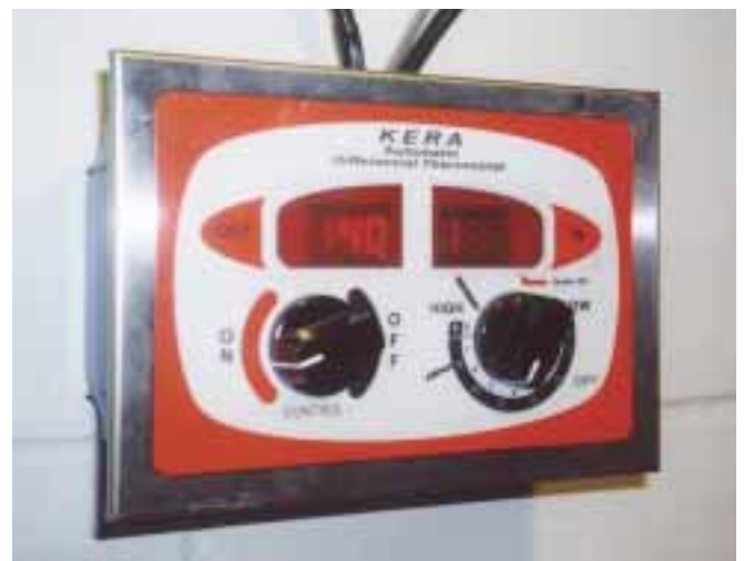
A Kera differential thermostat controls operation.
