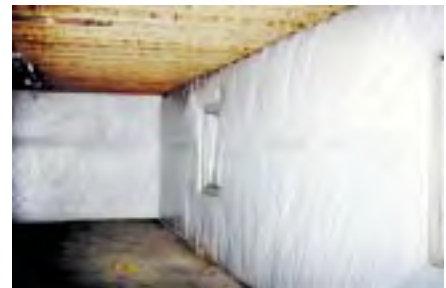
Photograph 3 Blanket insulation with impermeable vinyl interior surface
