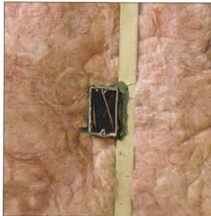
Details make all the difference. New Hampshire builder Doug George uses an 8-mil polyethylene air/vapor barrier on the warm side of the wall. The poly is caulked to framing members and electrical outlet boxes to prevent leaks.
