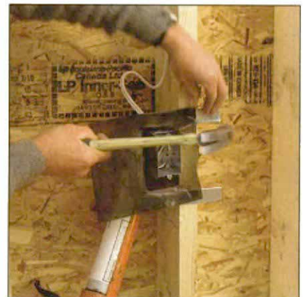
Sealing electrical boxes. An alternative method for sealing electrical boxes on outside walls is the "poly hat," which forms an air seal around receptacles. This technique is used by builder Peter Amerongen of Edmonton, Canada.
