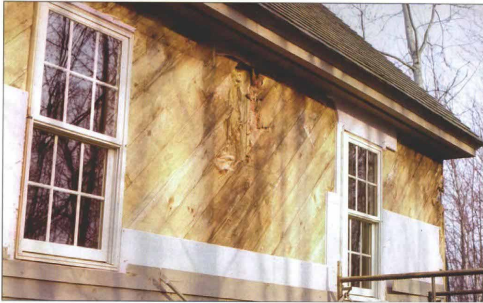
Moisture takes its toll. Sheathing and hemlock timbers in this Falmouth, Maine, house were so decayed in places that the wood could be pulled apart by hand. The apparent causes were high indoor humidity and a polyethylene air/vapor barrier that failed.
