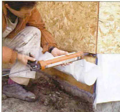
Sealing the rim joist. Builder Peter Amerongen devised an air-barrier technique that uses polyethylene on inside walls and strips of Tyvek housewrap to seal the rim joists. Acoustical caulk seals the top edge of the housewrap to the frame.
