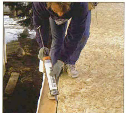
Second-floor rim-joist seal. To provide an air barrier at second-floor rim joists, Tyvek strips are sealed with acoustical caulk to top and bottom wall plates. Here, David Schuman puts a bead of acoustical caulk along the wall before it's raised into place.
