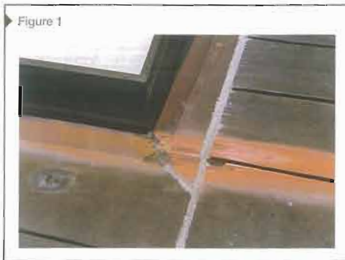
Figure 1 Corrosion occurred on this copper roof where condensation dripped from an aluminum skylight, while the remainder of the roof turned dark brown due to the influence of normal weathering. Images courtesy Simpson, Gumpertz, and Heger
