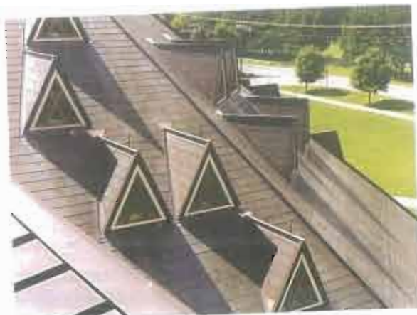
Many factors can affect the corrosion rate of metals on buildings, including rainfall, temperature, solar exposure, airborne pollutants, and even bird feces.
