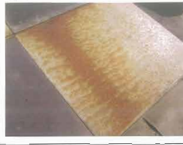
Copper over the aluminum/zinc-coated steel resulted in severe coating loss and rusting of the steel base.
