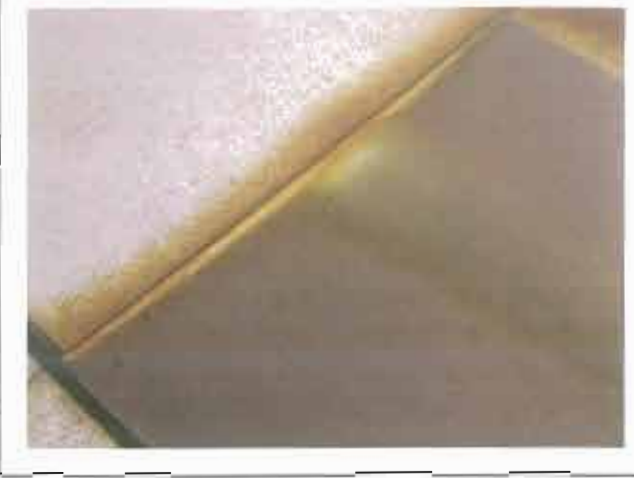
Corrosion product occurs within the lock between aluminum/zinc-coated steel and the copper.
