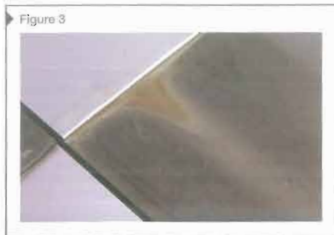
Figure 3 Runoff from stainless steel caused a portion of the copper panel to remain bright and shiny, indicating corrosion.
