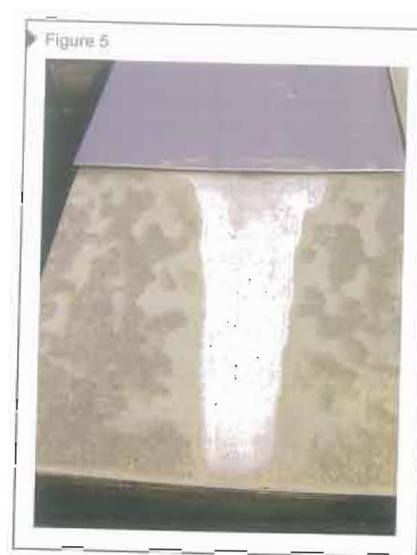
Figure 5 Stainless steel draining over tin/zinc-coated steel and copper caused white/gray staining on both pieces, indicating initial corrosion of the protective coating.
