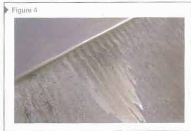
Figure 4 Stainless steel over lead-coated copper corroded portions of the lead. It caused staining and corrosion on most samples.
