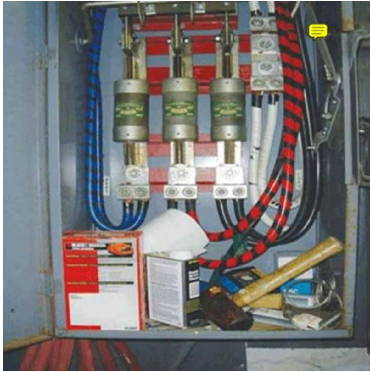
Main load, acetone, grits, and tool storage panel.
