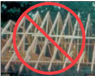
Above: Inadequate bracing - What Not To Do PHOTO B2-6
