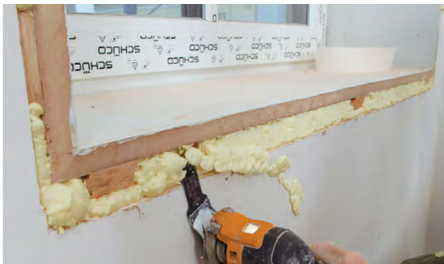
Cut back the foam. Use an oscillating multitool to cut back the excess spray foam after it cures to provide space for the drywall compound and paper tape.
