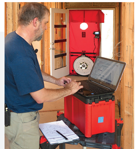
TEST THE SEAL. A professional blower-door test will identify any leaks you may have missed.
