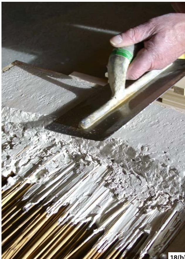
Figure 18: Bedding material being dressed with lime putty (a) over which, as in this demonstration, gypsum plaster is laid. (b) . Photos: Douglas D Kent (a) and AJ Goode Ltd(b)
