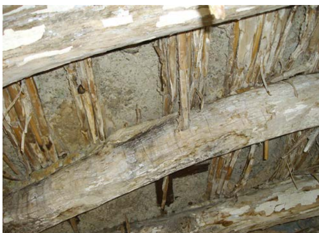
Figure 4: Cane bedding forming the underside of a historic gypsum plaster floor in Sierra, Andalucia, Spain.
