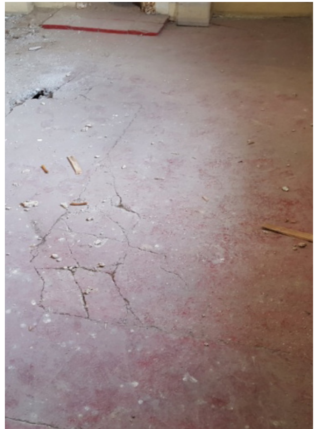
Figure 12: The nature and causes of defects should be clearly established before carrying out work involving an old gypsum plaster floor. Photo: Bonsers Restoration Ltd
