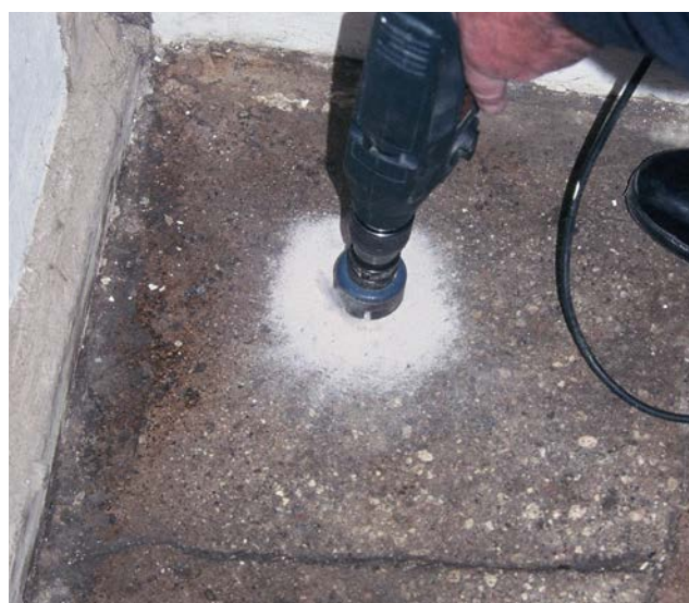
Figure 14: Drilling to remove a core sample of a gypsum plaster floor for laboratory analysis. Photo: A J Goode Ltd
