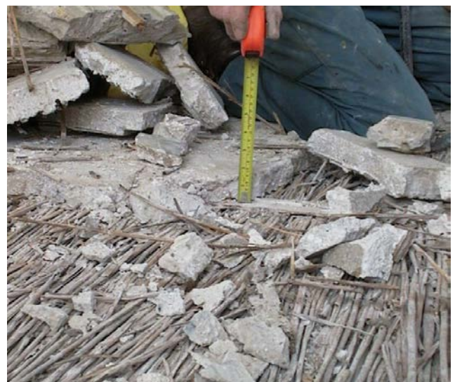
Figure 16: Old gypsum plaster that is removed should normally be retained for use as aggregate when laying replacement flooring. Photo A J Goode Ltd
