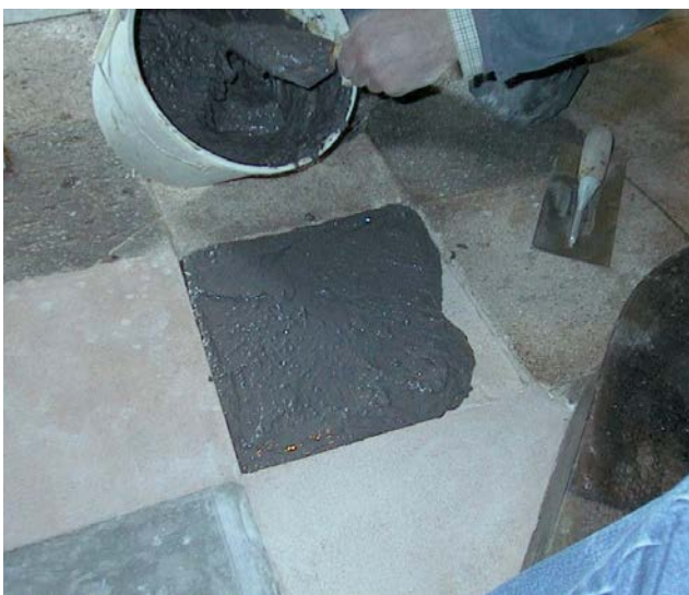
Figure 15: Materials and methods for repairs should match those of the original gypsum plaster floor as far as possible. Photo: A J Goode Ltd
