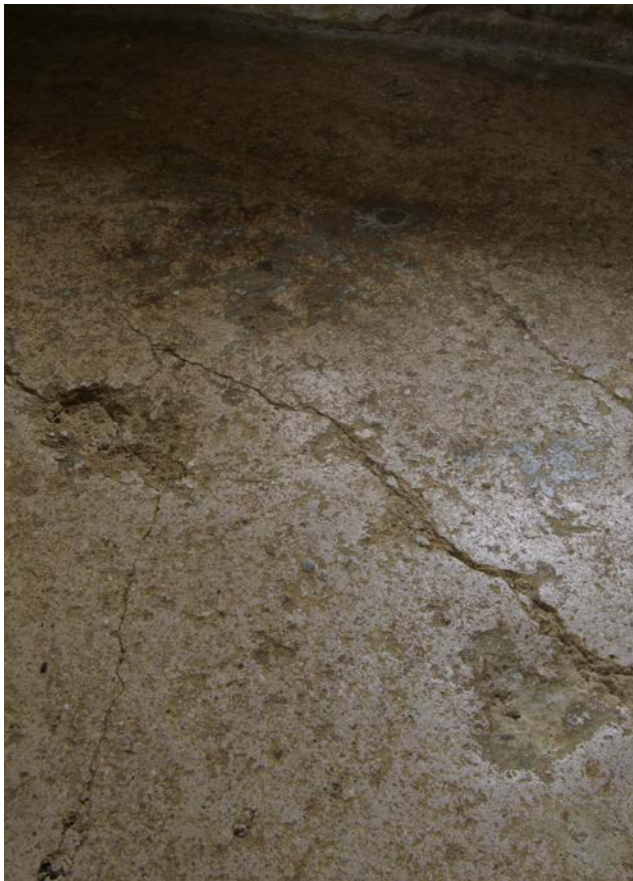
Figure 11: An old gypsum plaster floor may look beyond repair but can frequently be brought back into a sound, functioning condition. Photo: Douglas D Kent
