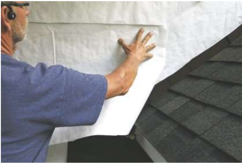
Slit the WRB and slide an additional piece of WRB into the slit to protect the square (black) piece installed earlier.
