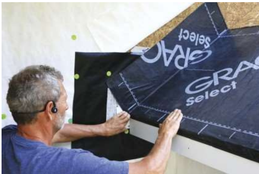
In cold climates, ice barrier laps over the fascia and up the wall.
