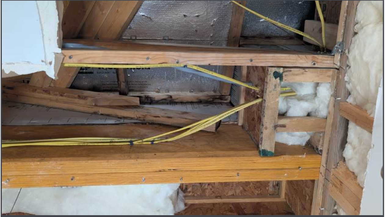
Garage attic radiant barrier. Horizontal beam at joint is point of water intrusion.
