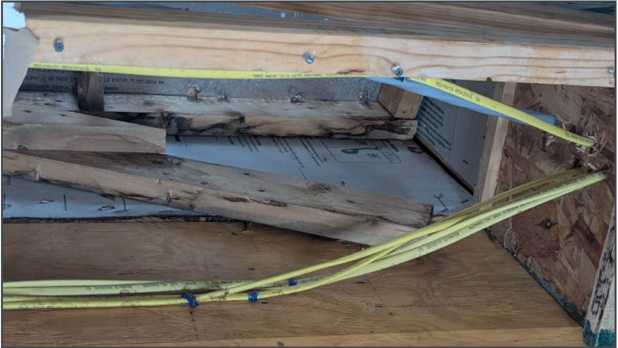
Horizontal beam at top of thermoply - point of water.
